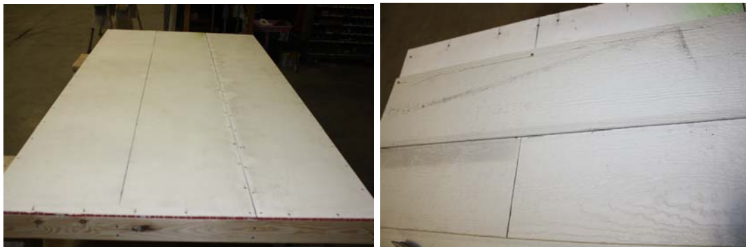
Test Series No. 1: Construction Photographs – Lap Siding (note butt joints every other course)
